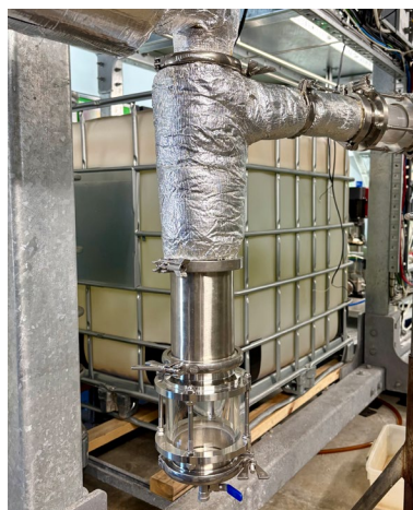
Uni-Dust Type 5 - Installed
